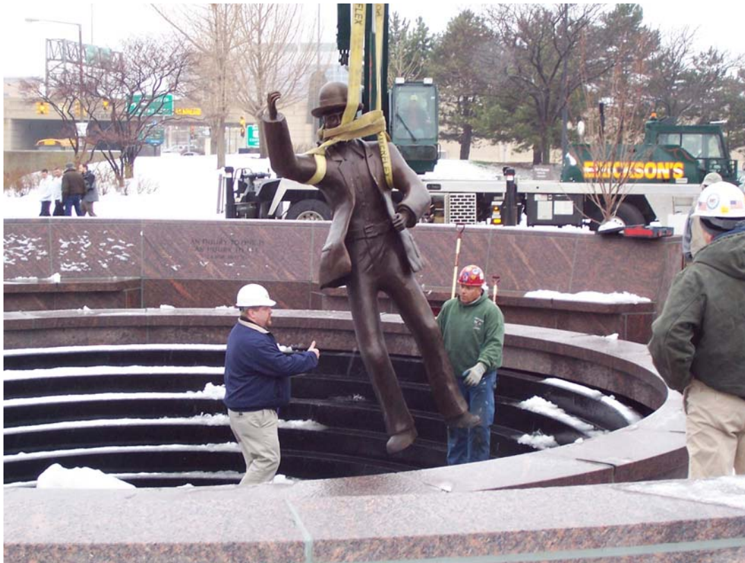
Mark Mangione, United Association Local 174 on the left and Tom Scheuneman, Ironworkers Local 340 are pictured setting the first figure on the granite base.
